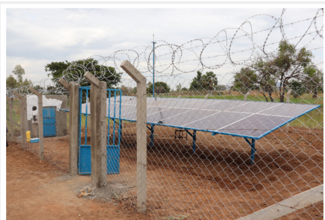
20 solar Panels with 265watts each
